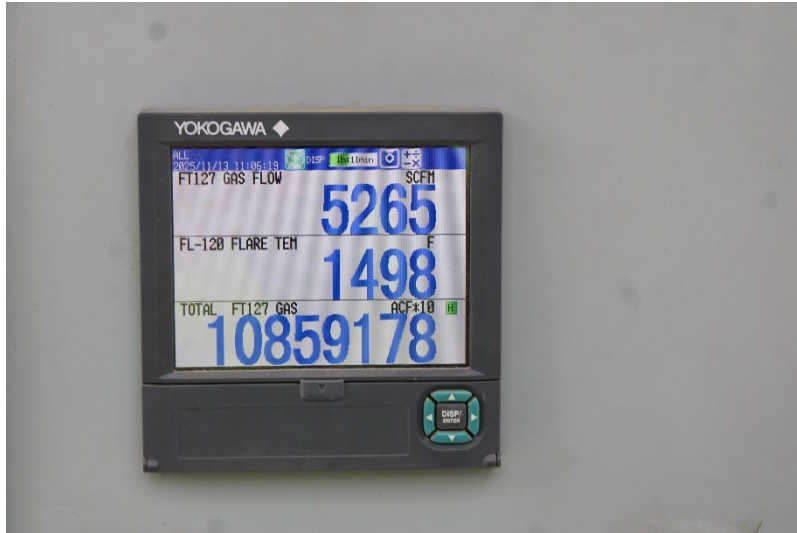
Photo 145: Flare 100, Flare 150 and Flare 250: November 13, 2025
