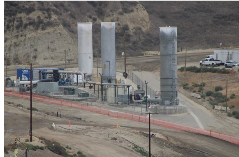
Photo 142: Flare 100, Flare 150 and Flare 250: November 13, 2025
