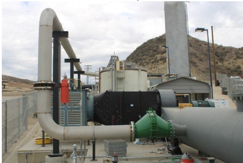
Photo 147: Flare 100, Flare 150 and Flare 250: November 13, 2025
