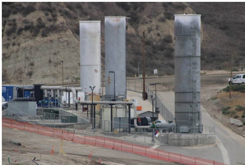
Photo 143: Flare 100, Flare 150 and Flare 250: November 13, 2025
