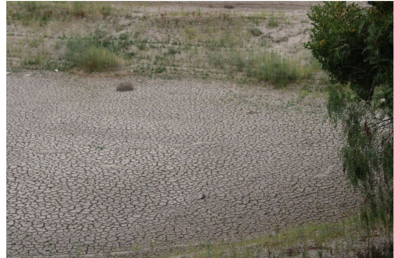
Photo 62: South Terminal and Catch Basins: July 22, 2025
