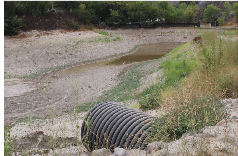
Photo 58: South Terminal and Catch Basins: July 22, 2025
