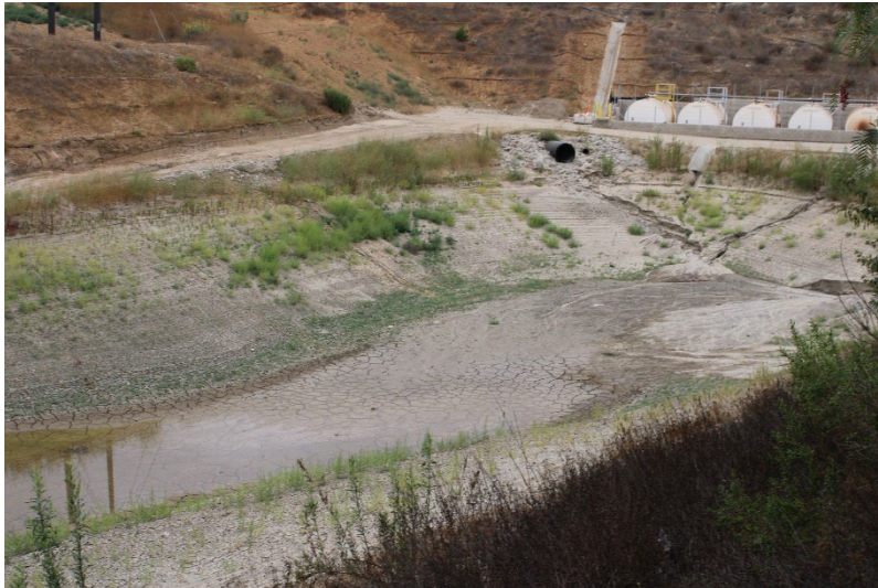
Photo 65: South Terminal and Catch Basins: July 22, 2025
