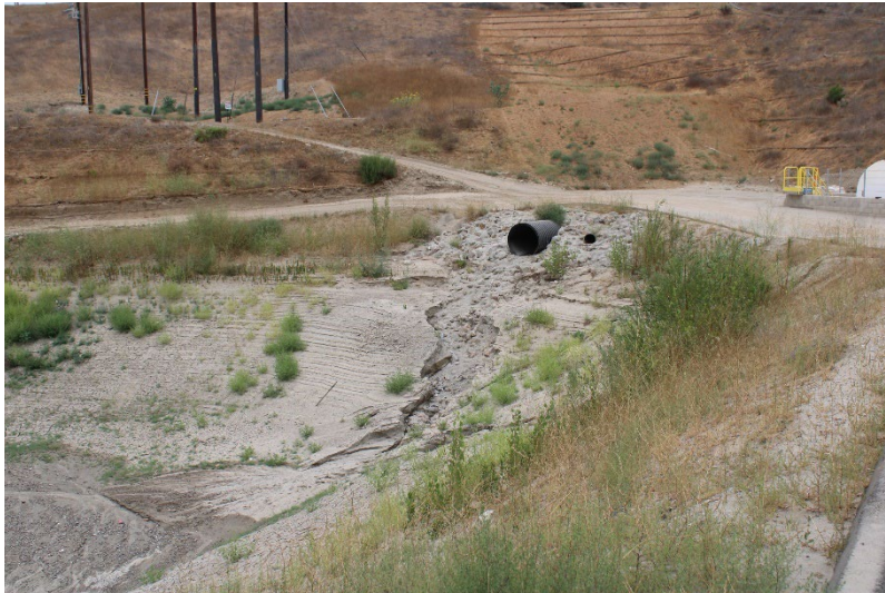
Photo 57: South Terminal and Catch Basins: July 22, 2025
