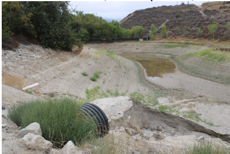
Photo 55: South Terminal and Catch Basins: July 22, 2025
