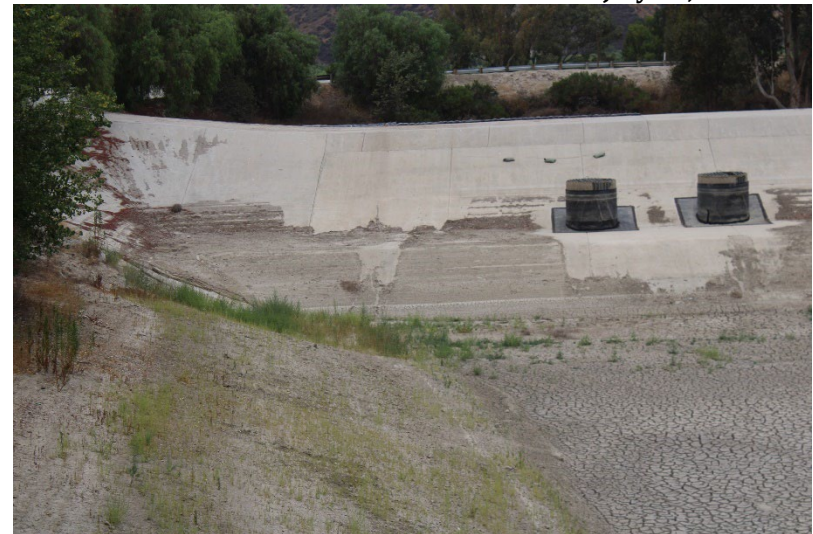
Photo 60: South Terminal and Catch Basins: July 22, 2025
