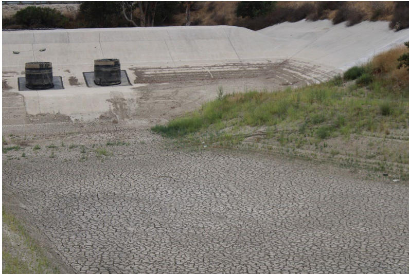
Photo 61: South Terminal and Catch Basins: July 22, 2025
