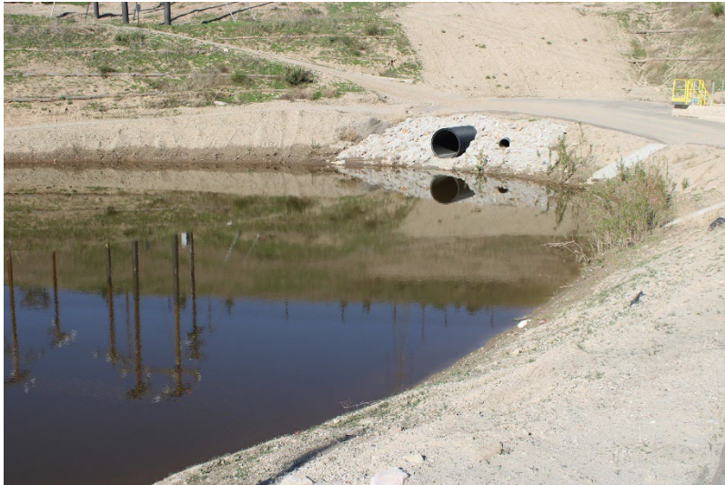
Photo 85: South Terminal and Catch Basins: March 20, 2025
