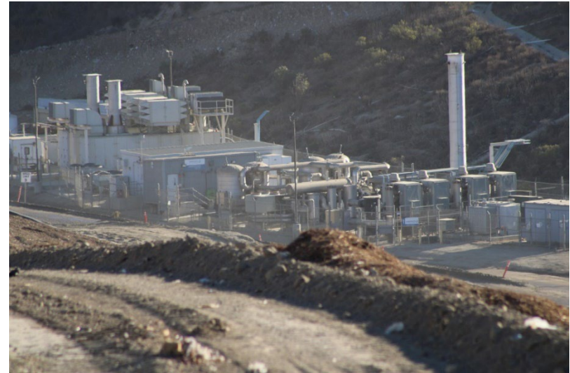
Photo 130: Gas-to-Energy Facility: January 16, 2025
