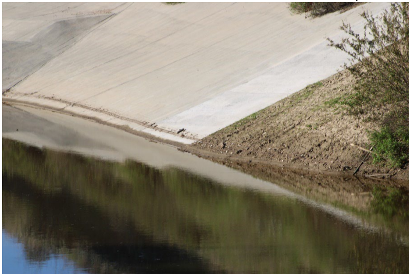
Photo 79: South Terminal and Catch Basins: March 20, 2025
