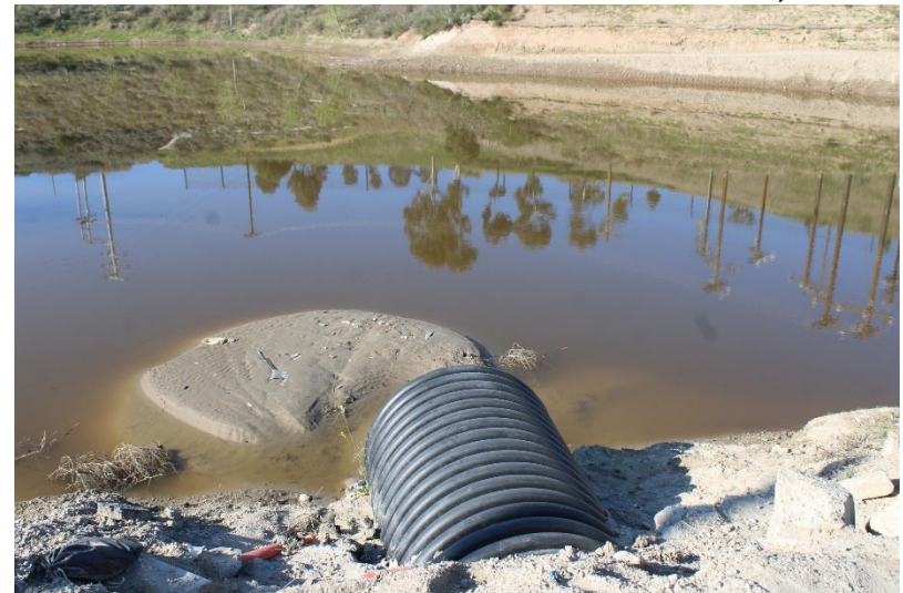
Photo 84: South Terminal and Catch Basins: March 20, 2025
