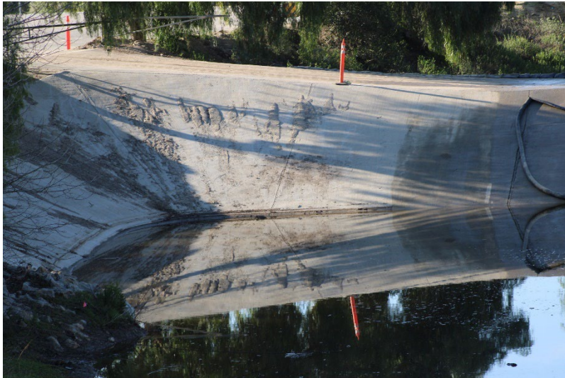
Photo 77: South Terminal and Catch Basins: March 20, 2025
