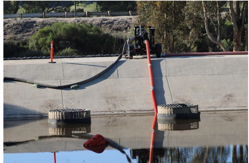
Photo 78: South Terminal and Catch Basins: March 20, 2025
