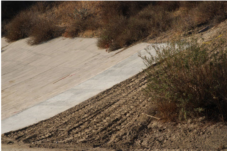
Photo 115: South Terminal and Catch Basins: December 3, 2024
