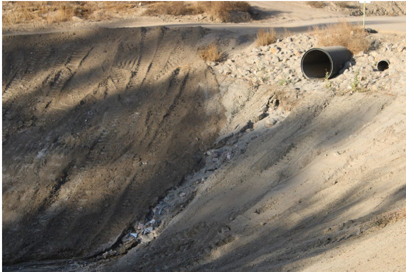
Photo 105: South Terminal and Catch Basins: December 3, 2024
