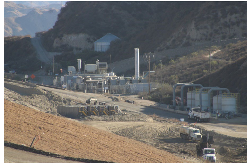
Photo 186: Gas-to-Energy Facility: October 23, 2024
