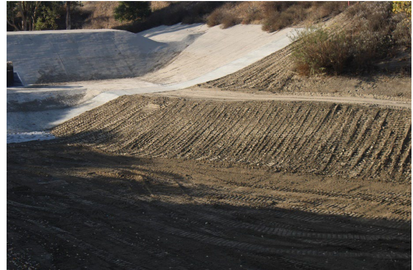
Photo 110: South Terminal and Catch Basins: December 3, 2024
