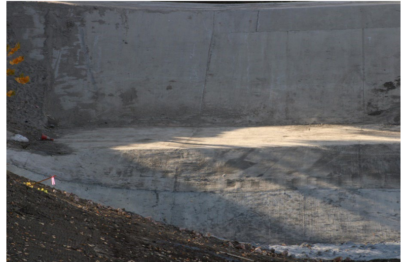
Photo 112: South Terminal and Catch Basins: December 3, 2024
