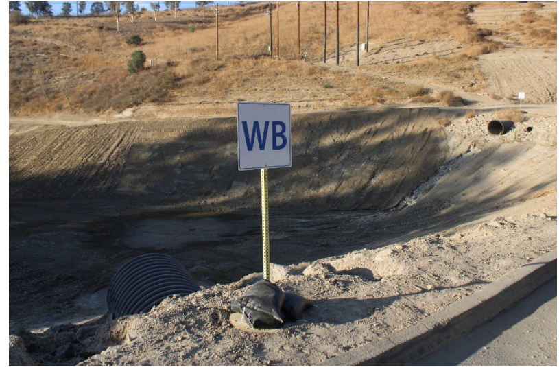
Photo 102: South Terminal and Catch Basins: December 3, 2024
