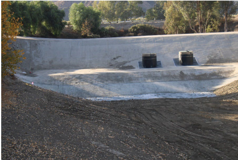
Photo 109: South Terminal and Catch Basins: December 3, 2024
