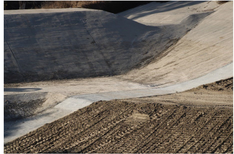
Photo 114: South Terminal and Catch Basins: December 3, 2024
