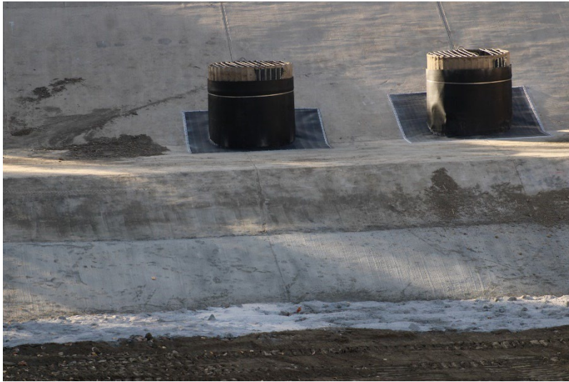
Photo 113: South Terminal and Catch Basins: December 3, 2024
