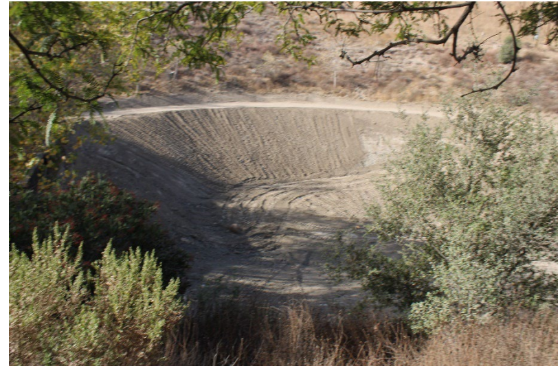
Photo 118: South Terminal and Catch Basins: December 3, 2024
