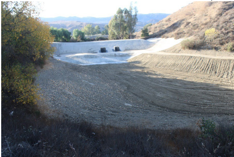
Photo 107: South Terminal and Catch Basins: December 3, 2024
