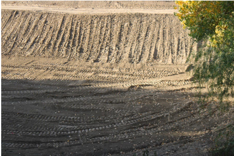
Photo 111: South Terminal and Catch Basins: December 3, 2024
