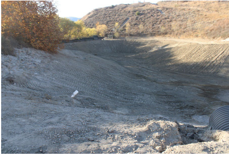
Photo 101: South Terminal and Catch Basins: December 3, 2024
