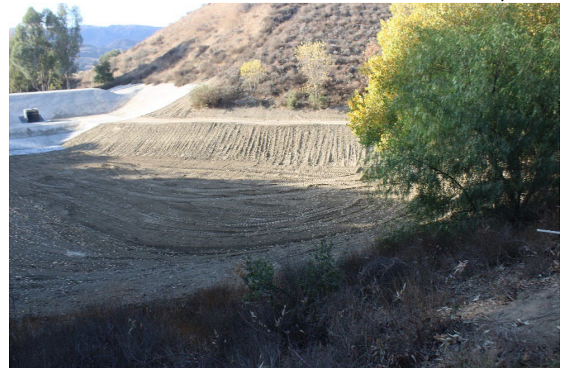
Photo 108: South Terminal and Catch Basins: December 3, 2024
