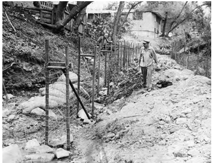
Figure 25. Kagel Canyon residents shoring up the canyon creek, 1962 (Los Angeles Public Library).
