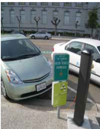
Example of an electric vehicle charging station.
