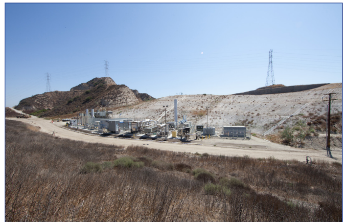
Gas-to-Energy Facility at the Chiquita Canyon Landfill
