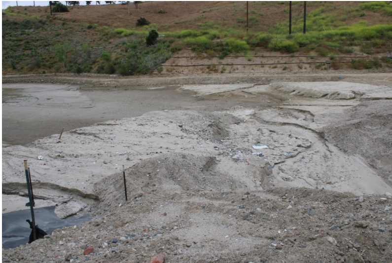
Photo 145: South Terminal and Catch Basins: May 25, 2023
