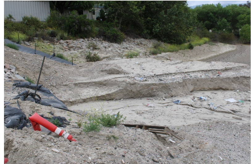
Photo 146: South Terminal and Catch Basins: May 25, 2023
