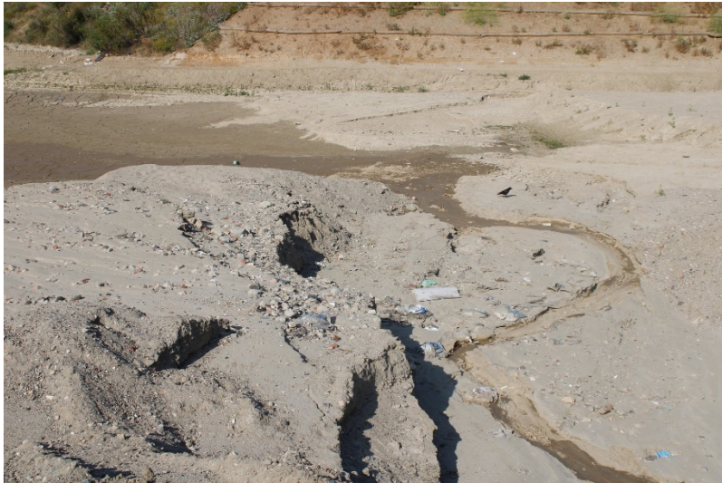
Photo 161: South Terminal and Catch Basins: June 14, 2023
