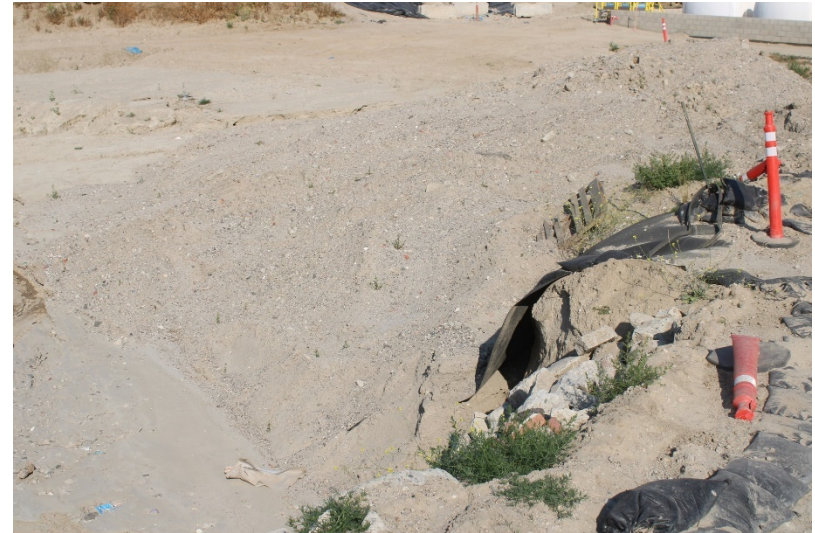
Photo 162: South Terminal and Catch Basins: June 14, 2023
