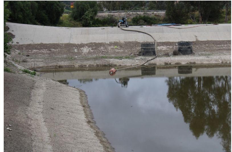
Photo 150: South Terminal and Catch Basins: May 25, 2023
