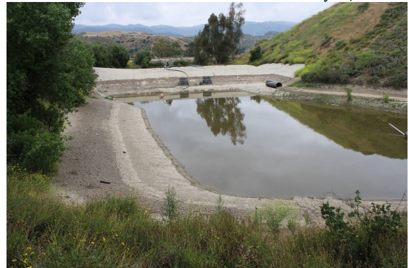
Photo 148: South Terminal and Catch Basins: May 25, 2023
