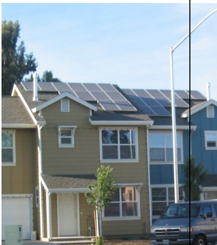
Example roof-mounted solar collector panels on multifamily housing.
