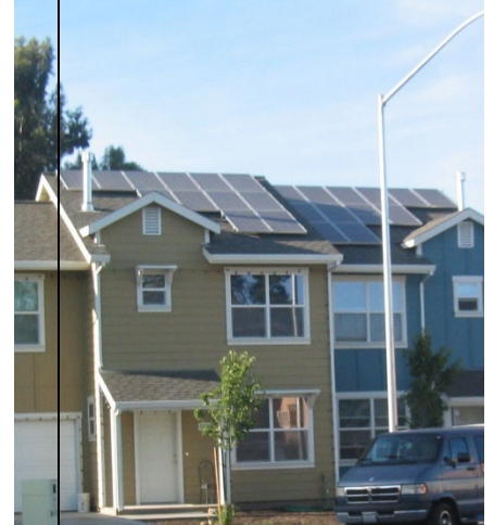
Example roof-mounted solar collector panels.
