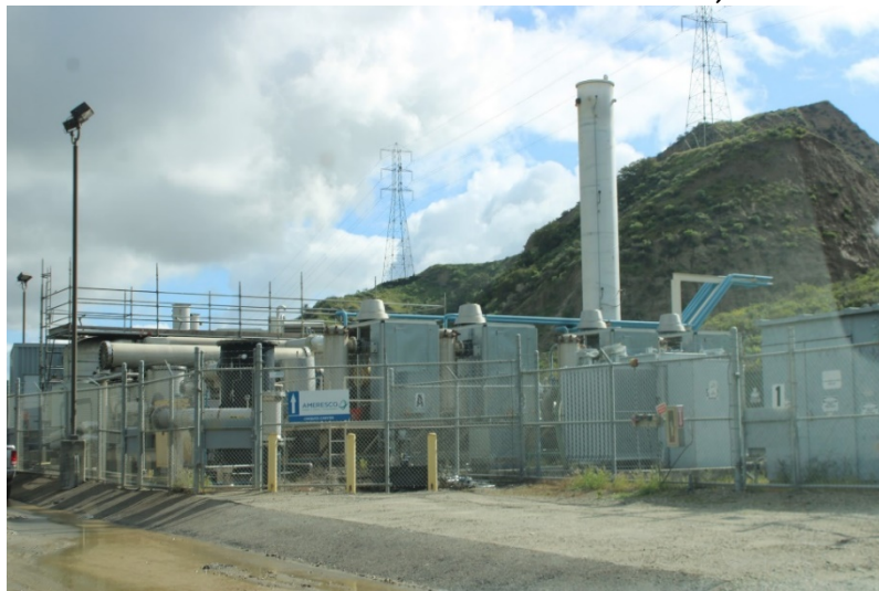
Photo 147: Gas-to-Energy Facility: March 23, 2023
