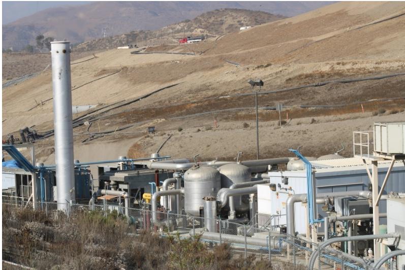
Photo 233: Gas-to-Energy Facility: October 12, 2022
