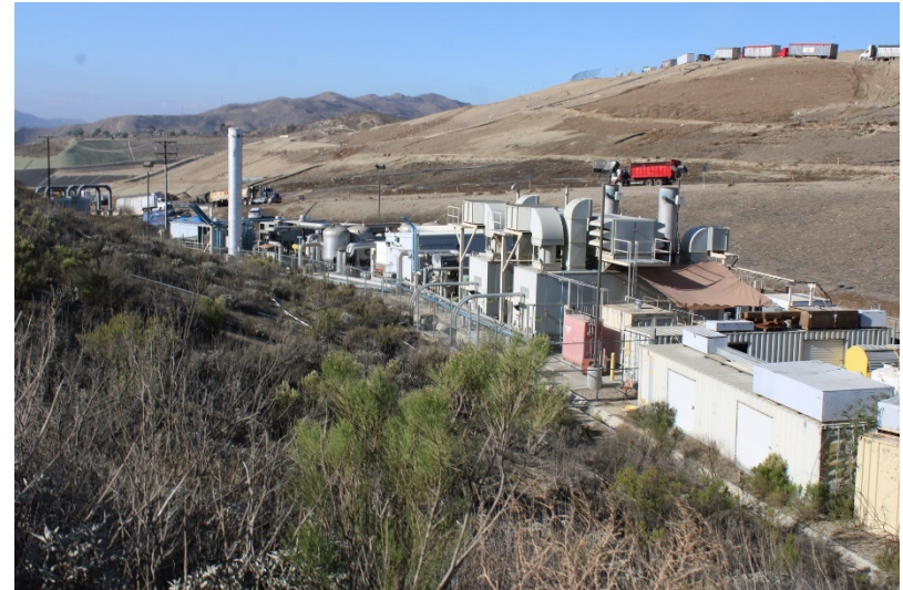
Photo 234: Gas-to-Energy Facility: November 30, 2022
