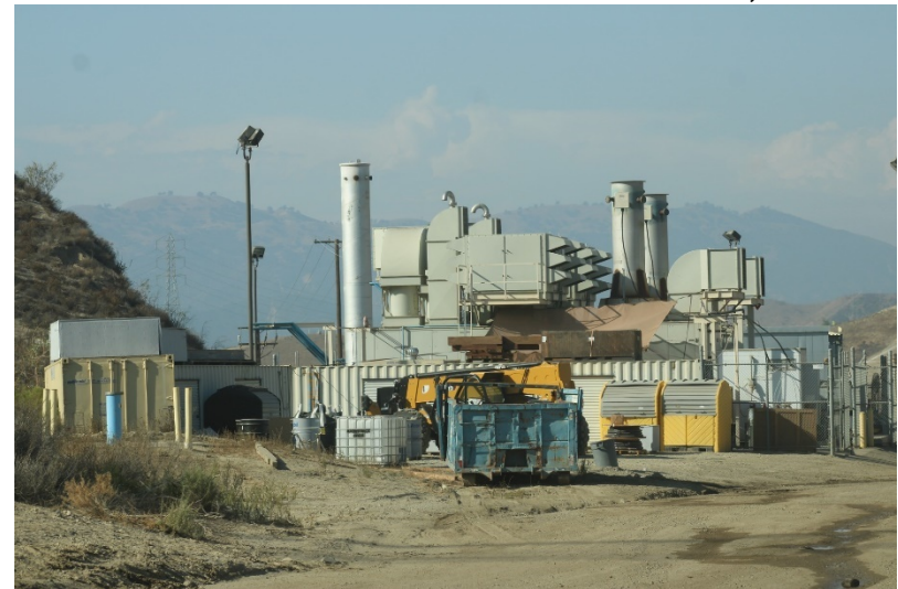
Photo 232: Gas-to-Energy Facility: October 12, 2022
