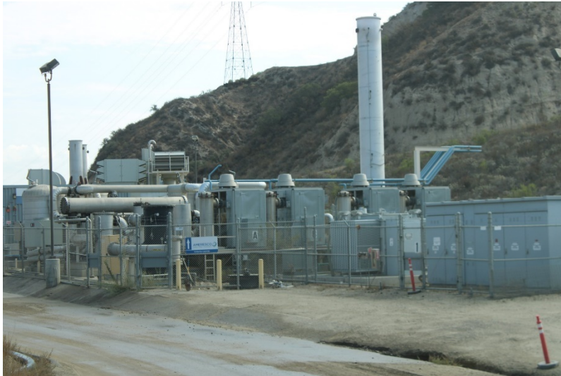
Photo 265: Gas-to-Energy Facility: September 13, 2022
