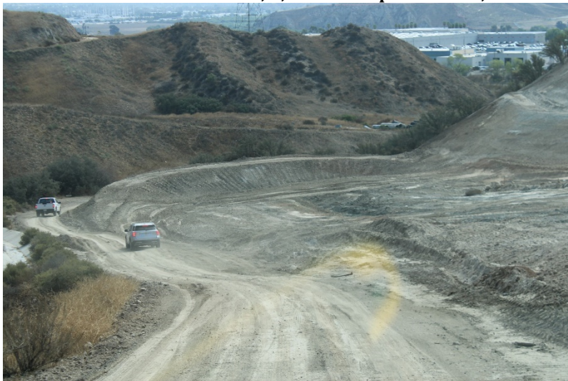
Photo 155: Future Cells 7, 9, and 10: September 13, 2022
