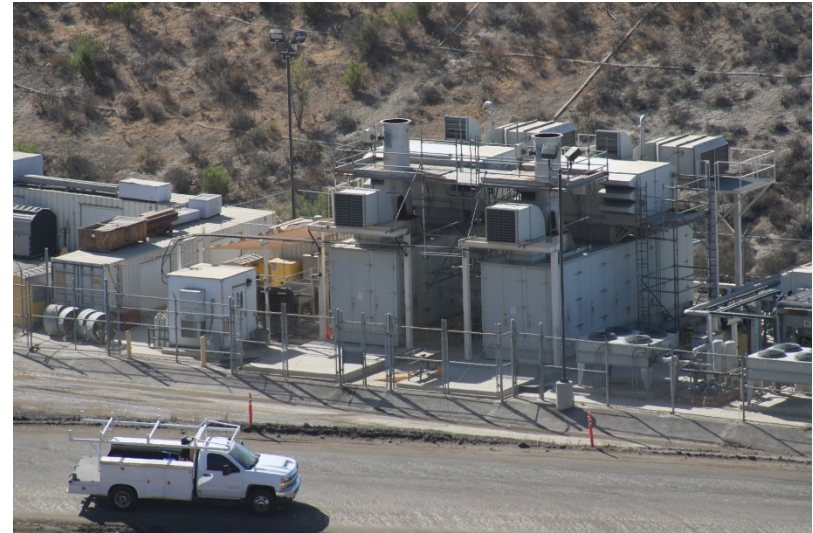
Photo 262: Gas-to-Energy Facility: July 21, 2022
