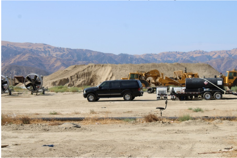
Photo 127: Closed Landfill - Primary Canyon: September 13, 2022
