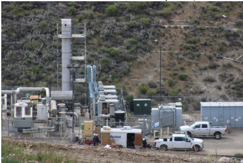
Photo 259: Gas-to-Energy Facility: April 26, 2022
