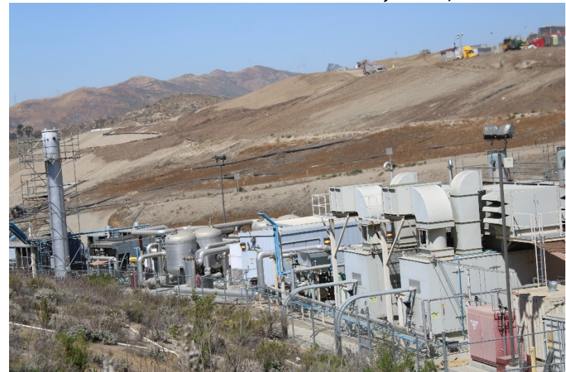
Photo 260: Gas-to-Energy Facility: May 24, 2022
