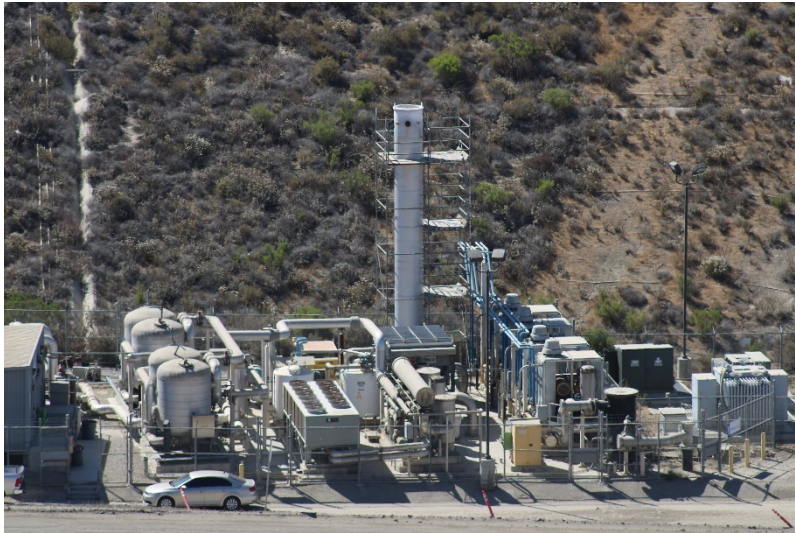
Photo 261: Gas-to-Energy Facility: June 21, 2022
