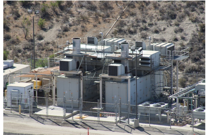
Photo 261: Gas-to-Energy Facility: June 21, 2022
