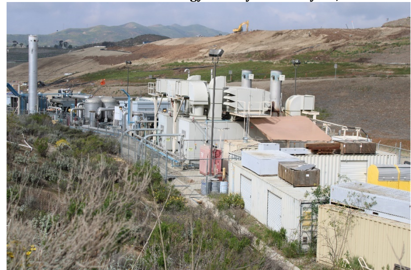
Photo 184: Gas-to-Energy Facility: March 31, 2022
