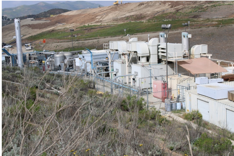
Photo 185: Gas-to-Energy Facility: March 31, 2022
