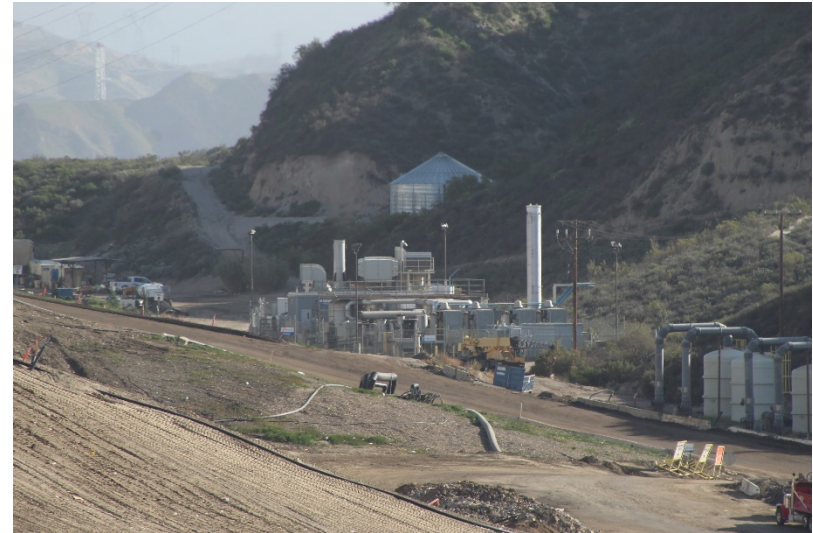
Photo 182: Gas-to-Energy Facility: February 22, 2022
