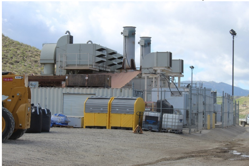
Photo 183: Gas-to-Energy Facility: February 22, 2022
