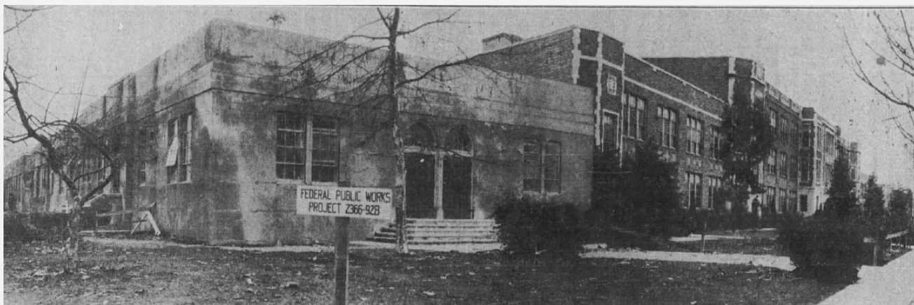
Exhibit 16. Thomas A. Edison Junior High School during reconstruction and redesign work after the 1933 Long Beach earthquake, 1935
