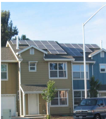
Example roof-mounted solar collector panels.
